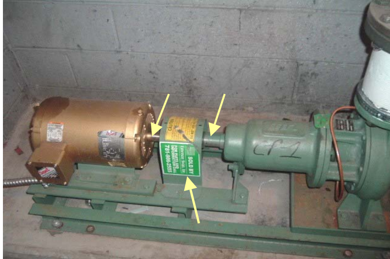
An inadequate guard on a small heating system pump. The shaft is exposed on both the motor and pump sides of the coupling.
